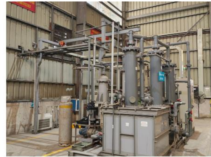
Destruction facility in Vietnam
